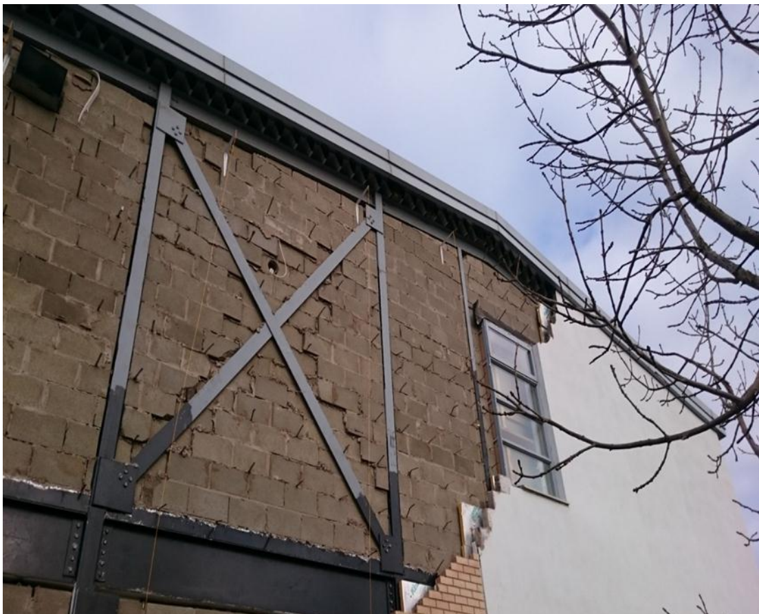
Image 5: Photograph of exposed inner blockwork leaf of gable after removal of insulation demonstrating the recessed blockwork in the braced bay which resulted in extending the width of the cavity.
