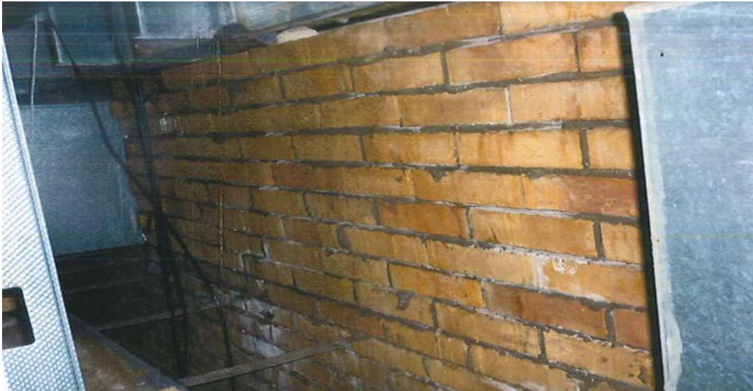
Image 27: Photograph from Duncanrig Secondary School. 'Note no ties or head restraints to inner face of outer brick leaf'.
