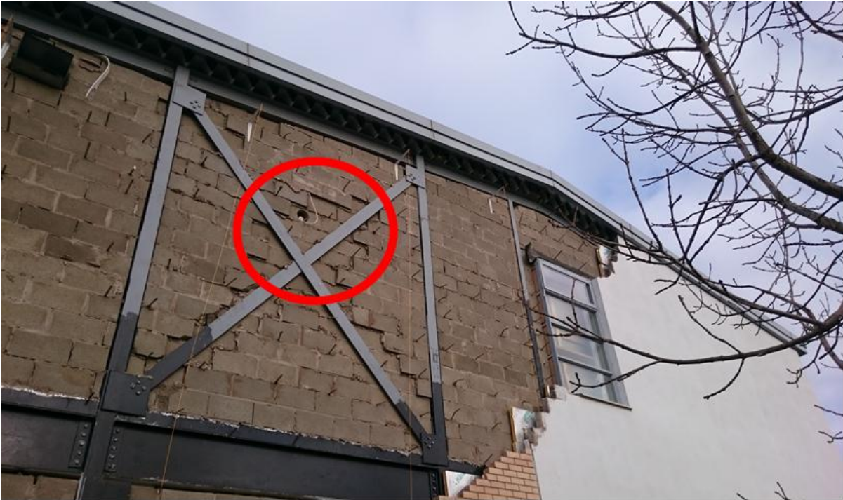
Image 23: Photograph of the collapsed section of the Oxfangs gable wall.
