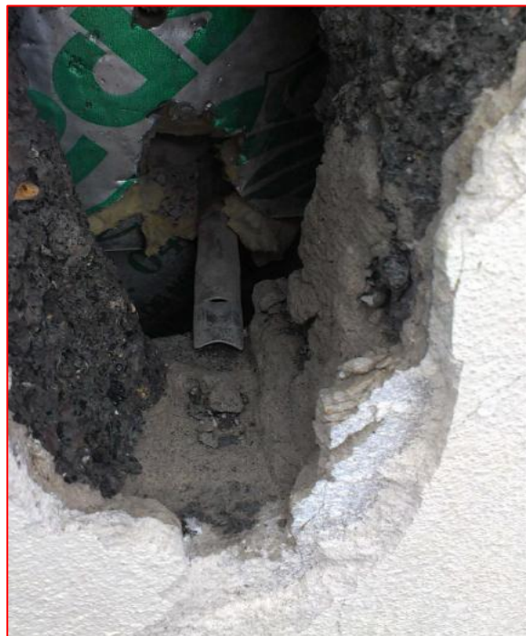
Image 9: Photograph from the survey reports. This photograph shows very limited embedment of a wall tie at Forthview Primary School.
