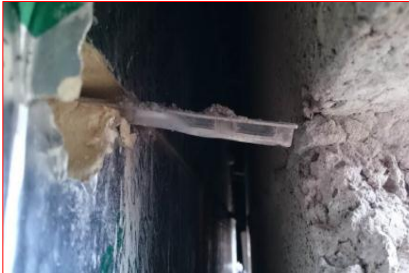
Image 8: Photograph from the survey reports showing the lack of embedment. This is an example of no embedment of a wall tie at Howdenhall Centre.
