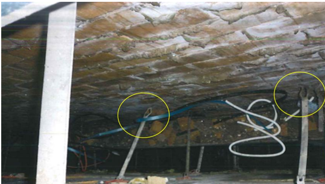
Image 28: Photograph from Duncanrig Secondary School. 'Note wall ties with no embedment in outer brick leaf of cavity wall'.
