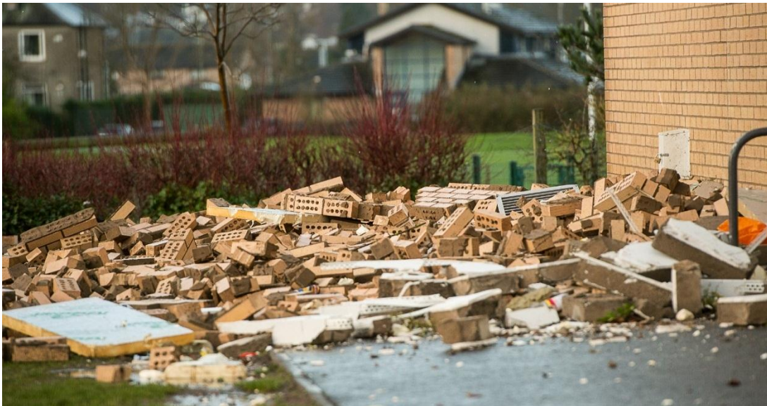
Image 3: Photograph taken at Oxgangs School of the gable wall after the collapse.
