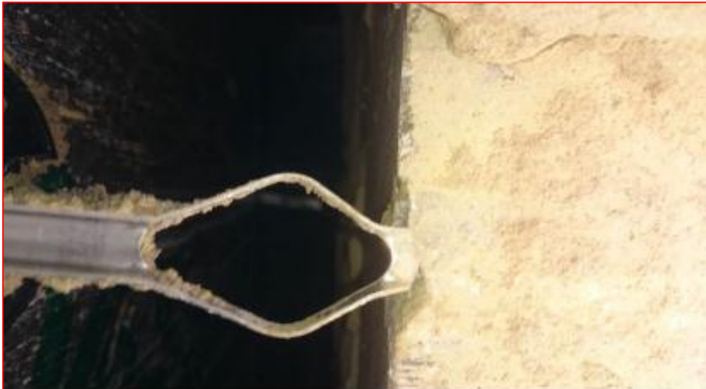
Photo 0185 Location 61A – Embedment 0mm
