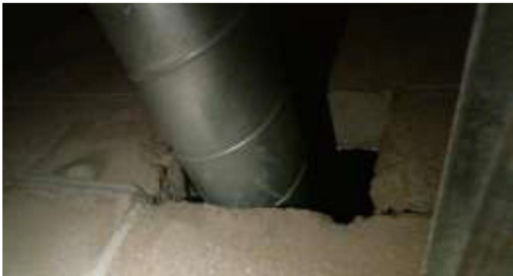
Image 22: Example of a breach of fire compartmentation from the fire-stopping survey of Royal High School, dated 22 nd August 2016 : "the pipe has not been fire stopped and a breach exists."
