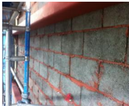
Image 30: St Ninian's High School; "No wall ties have been installed into a large section of the wall."
